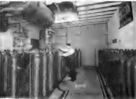
The Eisler hydrogen and oxygen tank room supplied the automatic lead-in wire plant in 1926.
